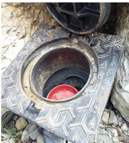
Photo 7: captage rate aval, regard siphoné
